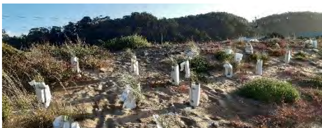
Sand placed over rock revetment and planted out with native coastal species and a section of the stabilised bank around 9 months later.
